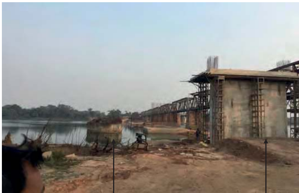
Figure 3.10: Abandoned bridge constructed with Well foundation New bridge constructed with Pile foundation
